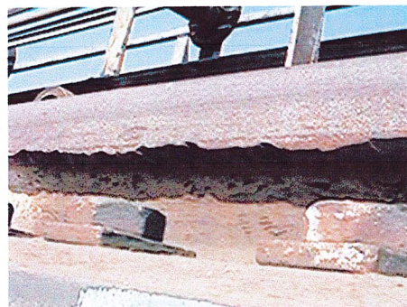
Figure 9: Erection defects – Case 3.
